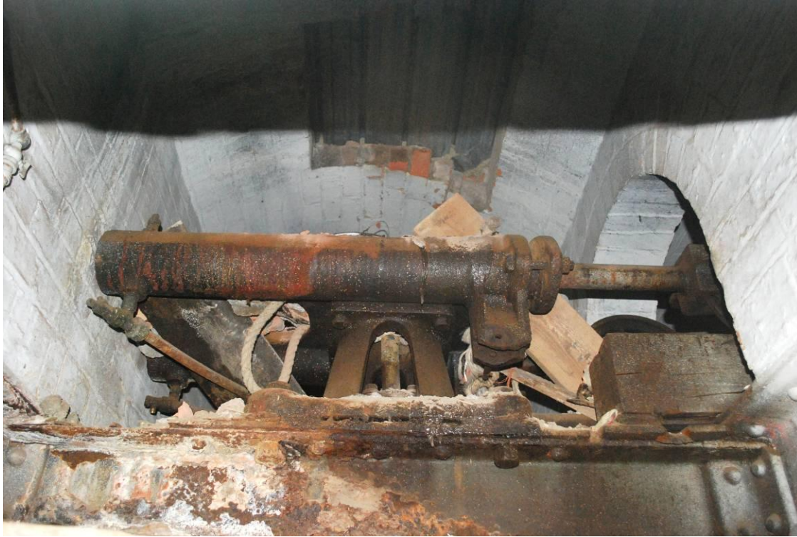
Fig. 31 (above): Slewing cylinder mounted on bottom support for crane, remaining in situ at C/D-14, viewed from east. Compare Fig. 25.
