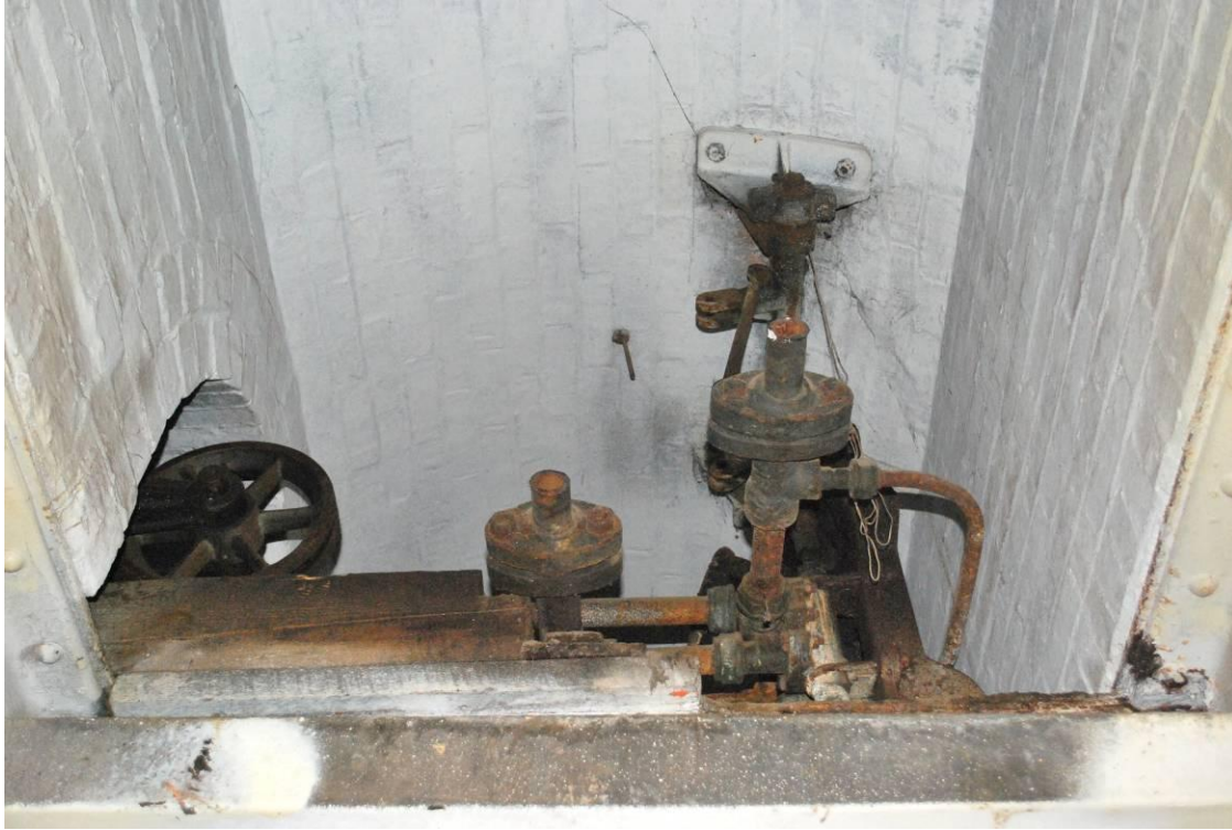
Fig. 33 (above): View of next ceiling bay, showing pulley on slewing ram protruding through archway, and control gear on right. Note hydraulic pipework, severed at front. View from east.
