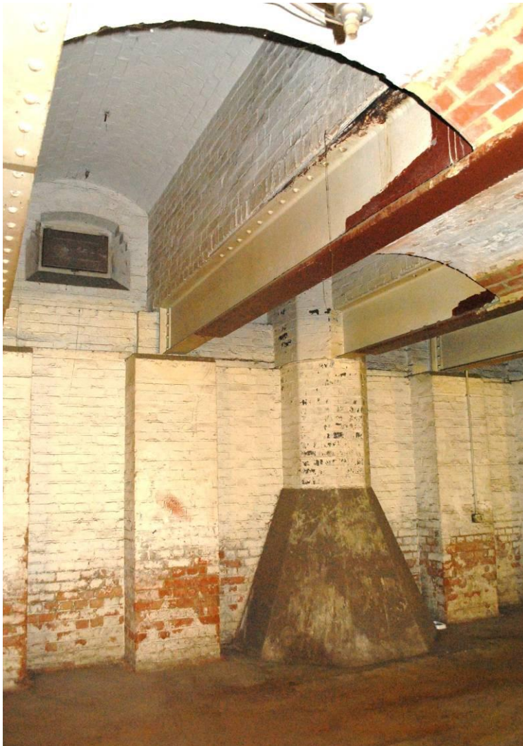
Fig. 20: Dividing wall between Basement and Dock, with flared column base and ventilation shutter. View from SE.
