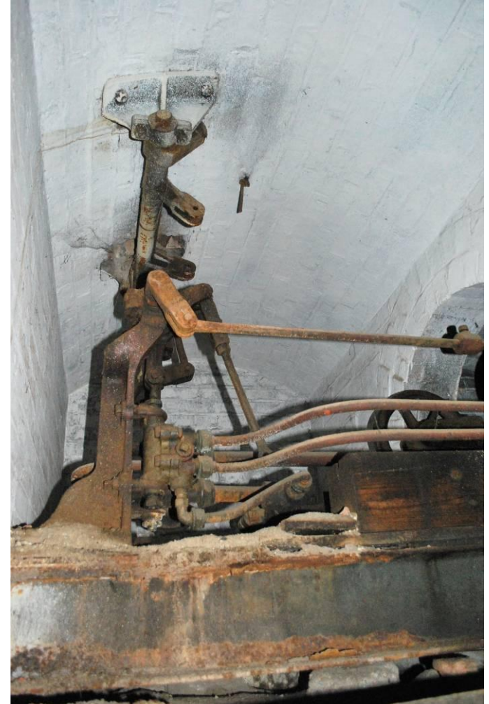
Fig. 34 (right): View of control gear from west. Note fixing brackets on ceiling, which are next to two holes for control rods or cables.
