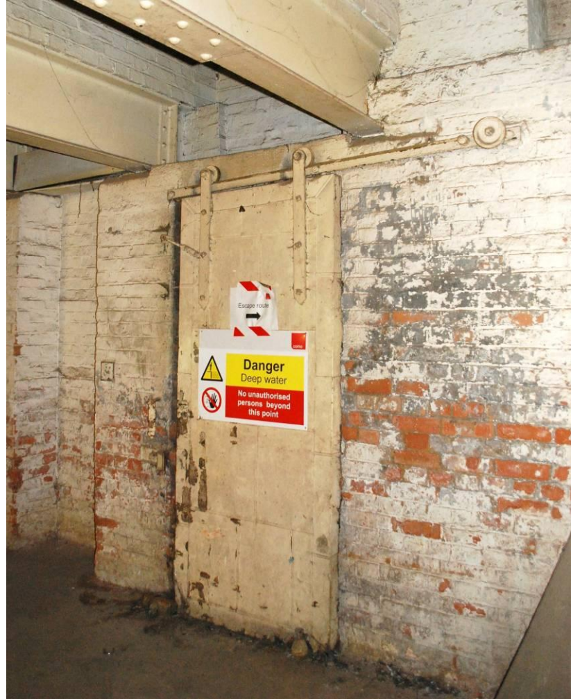
Fig. 36: Sliding Fire Door to Dock at D-13/14
