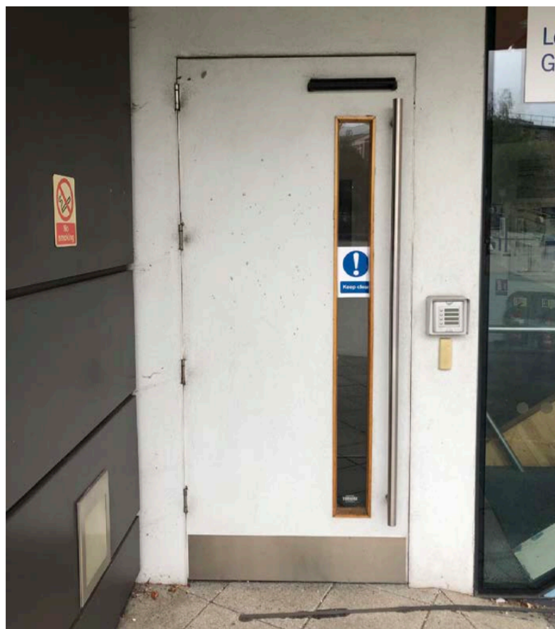
Existing entrance to be door to be replaced
