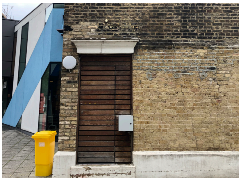
Brickwork to be cleaned, repaired and repointed
