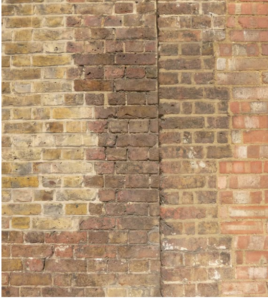
Fig. 11: Patchwork repairs to the Victorian building
