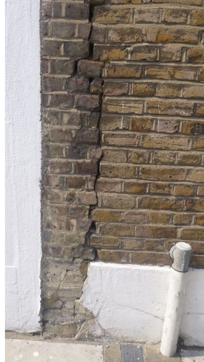
Fig. 18: Poor quality construction of 1965 building
