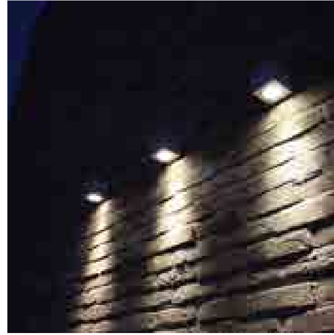
M42 External lighting
