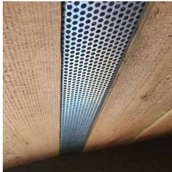
M25 MVHR supply and extract within the brick soffit of window reveals
