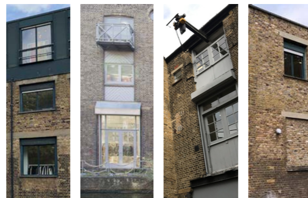
ref 2.36 Photographs and typical windows for Regents canal buildings and Eagle Mews
