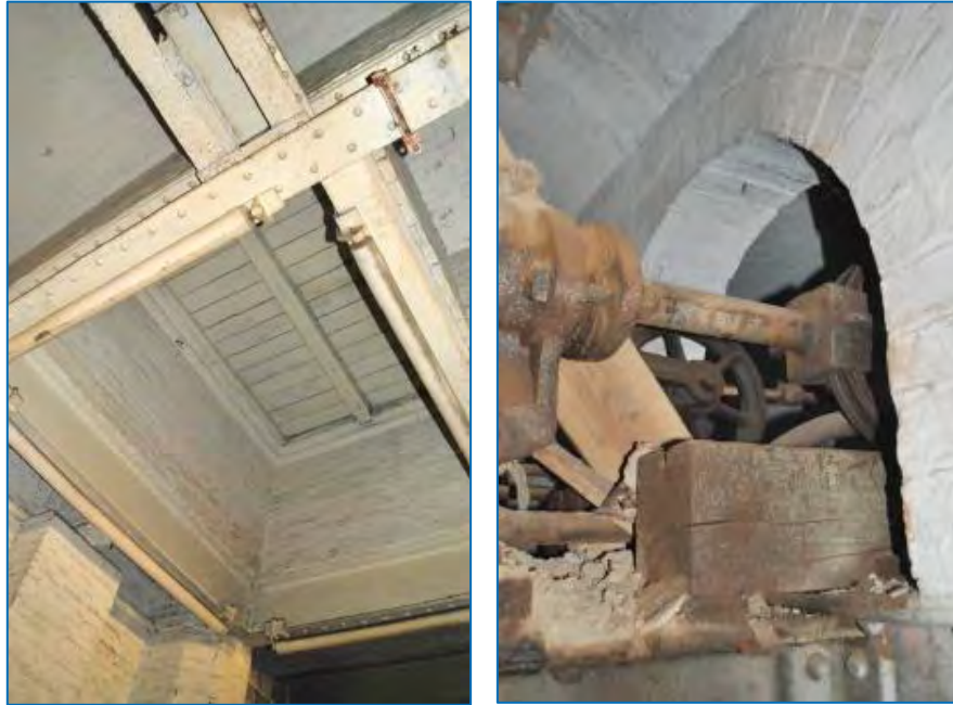
Figure 4.14: Trap door in platform above basement (left) Slewing Rams extending through the archway (right) 49
