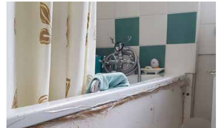
Fittings and fixtures have reached their end of life
