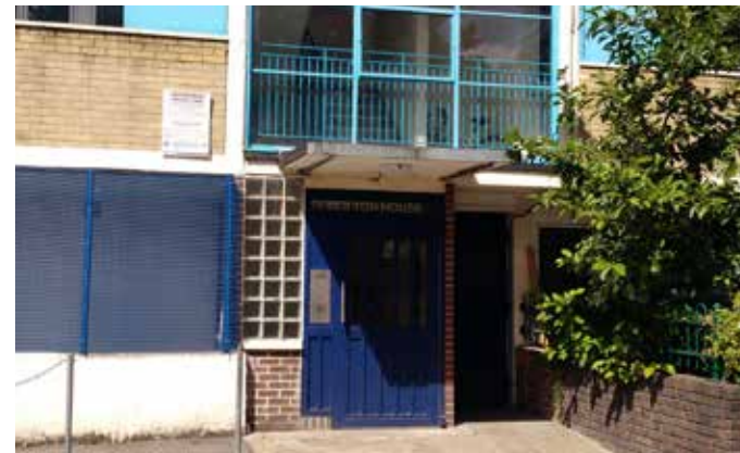
Uninviting, unsafe, poorly lit entrances
