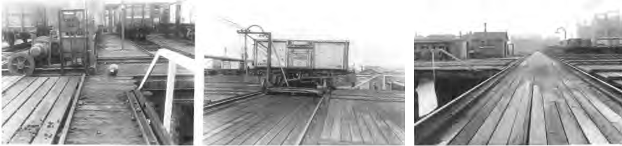
Figs 10-12: The Plimsoll Viaduct Bridge over the Regents Canal to The Cambridge Street (formerly Plimsoll) Coal Depot
