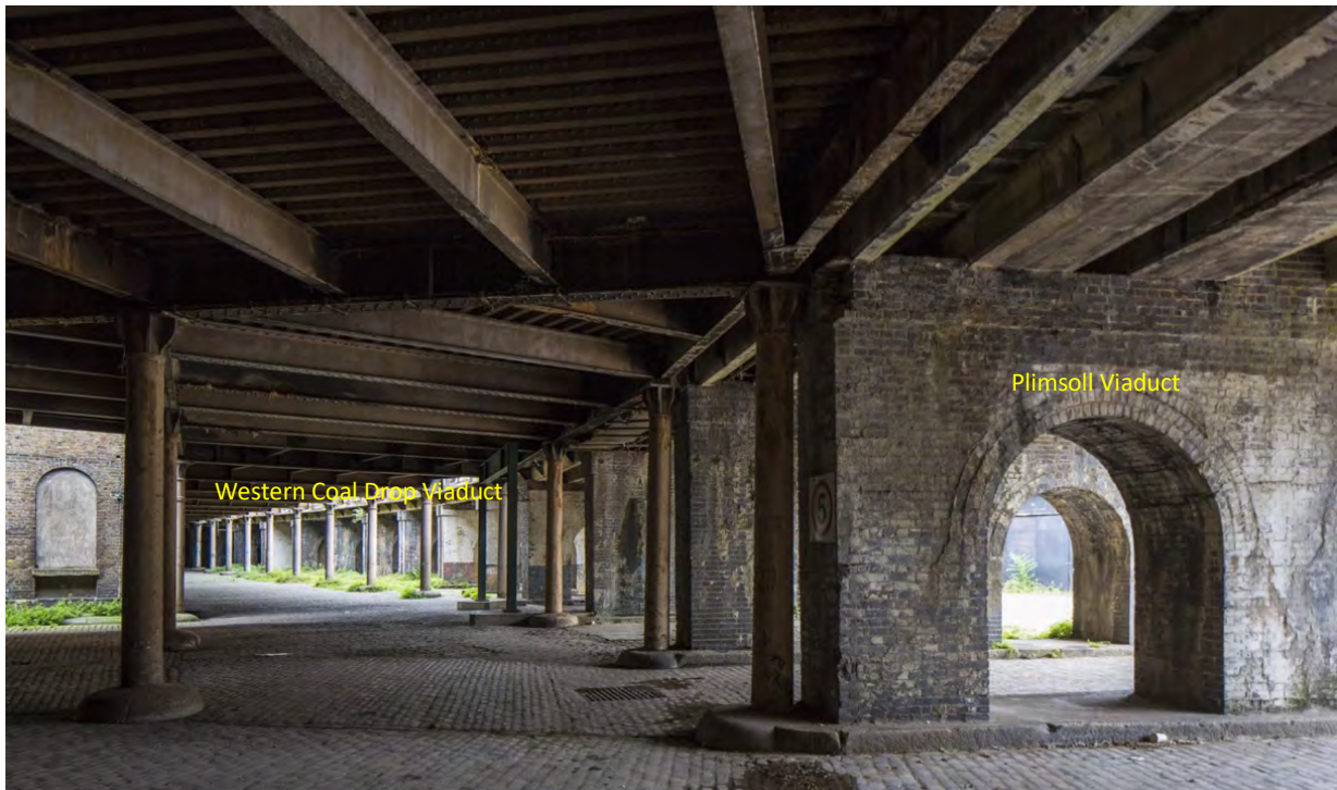
Fig 16: The Western Coal Drop Viaduct (l) and rebuilt Plimsoll Viaduct (r) looking north from the Wharf Road abutment prior to the removal of the Plimsoll Viaduct in 2012. The Cast Iron Western Coal Drop Viaduct dates from 1857 when it was originally located on the western side. It was relocated to the eastern side and extended to the south in 1897 as a road viaduct. The Plimsoll Viaduct was rebuilt in the 1920s in blue engineering brick and reinforced concrete. It was removed to better reveal the earlier Western Viaduct and to enable north south circulation through the Yard.
